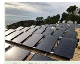
350 m 2 covered PV collectors in Spain.
